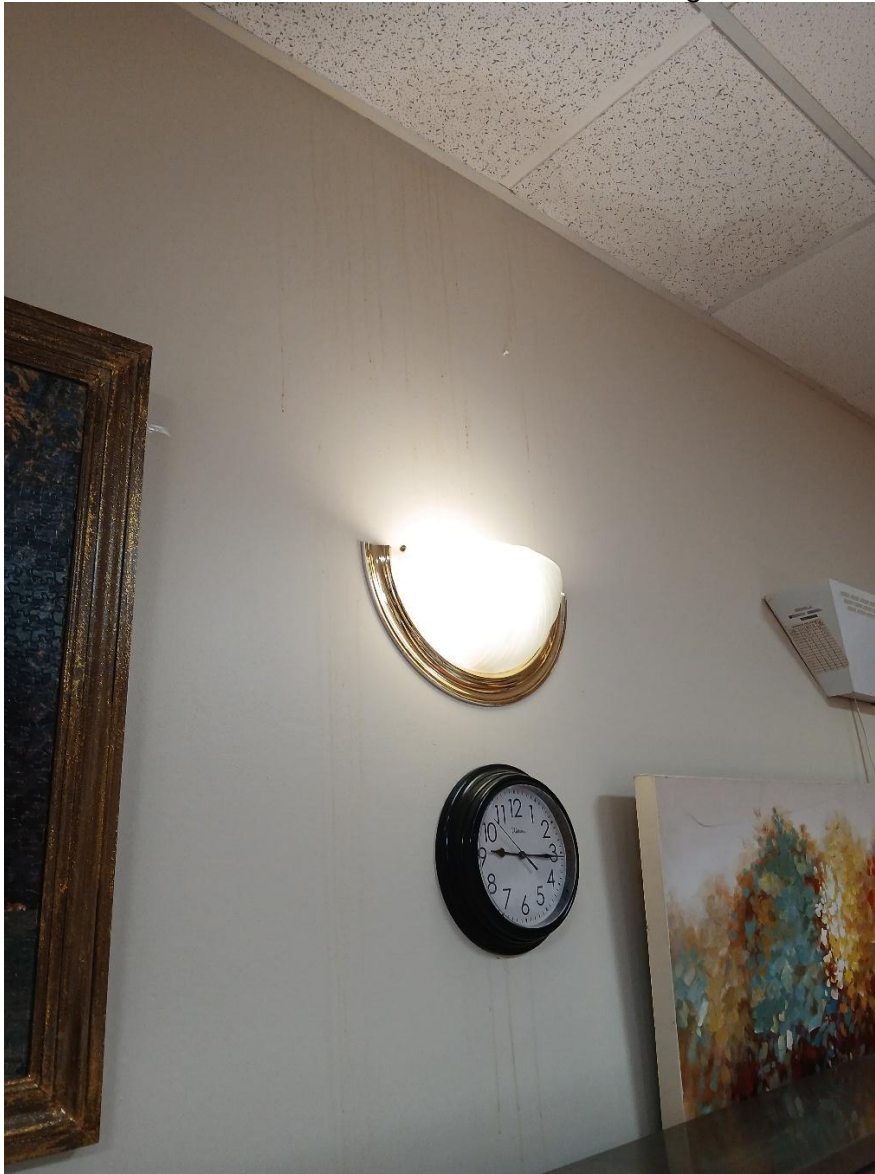
Photo taken 3/23/2026 2 nd floor, water running down wall in hall
