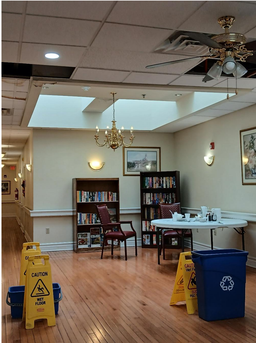
2 nd Floor ceiling leak and buckets
